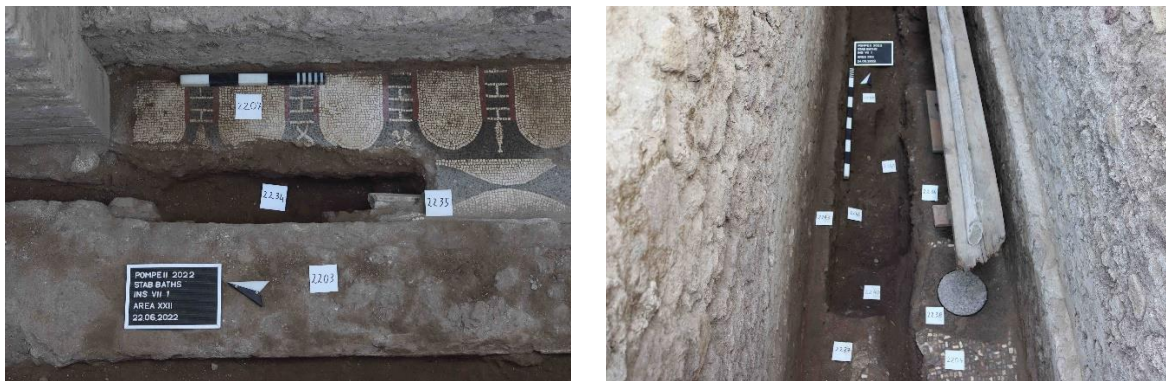
Fig. 14: Area XXII, corridor H': lead pipes of the house (phase 2) and baths (phase 4b)
